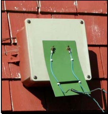
Figure 10 – Strain relief on the transmitter end. Inside the PVC box are threaded ¼” steel rods in PVC pipe going through the wall to the tuner.
